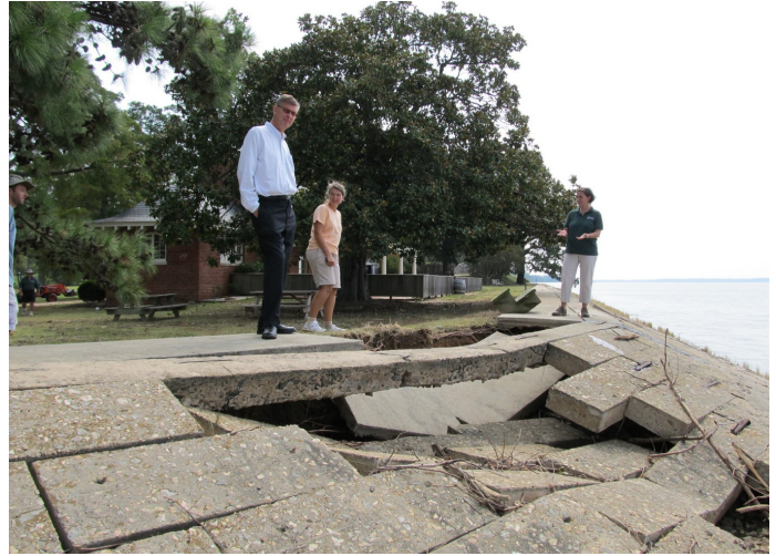
Hurricane Irene damage in 2011.
