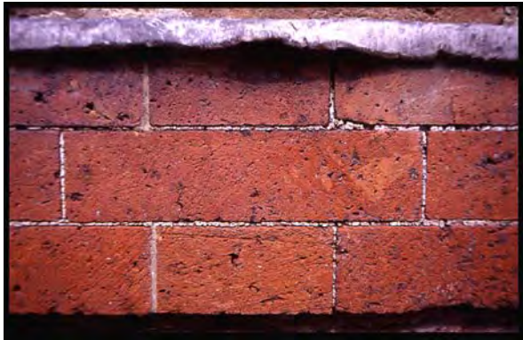
Detail of the stringcourse at the College of William and Mary (1695-1697). Mortar joints average 3/32". The lead capping, which is largely original, was originally painted red. Photograph by Willie Graham, 2001.
