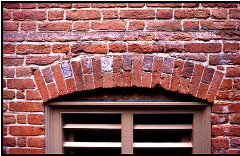
College of William and Mary, Williamsburg, Virginia. The brick walls were laid between 1695 and 1697. Although lightly glazed bricks have been randomly dispersed throughout the walls, headers have been deliberately picked out in the cellar arches. Note that the water table and the course below it have been rubbed. Photograph by Willie Graham, 2001.
