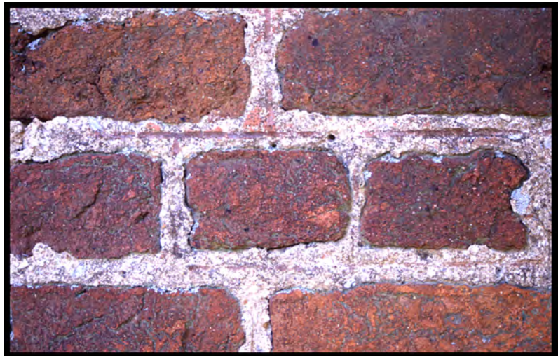
Detail of painted mortar joints and brickwork at Bacon's Castle (1665) in Surry County, Virginia. Paint analysis by Susan Buck revealed that the masonry was given a red wash from the outset, before the mortar had time to cure. Photograph by Willie Graham, 2002.
