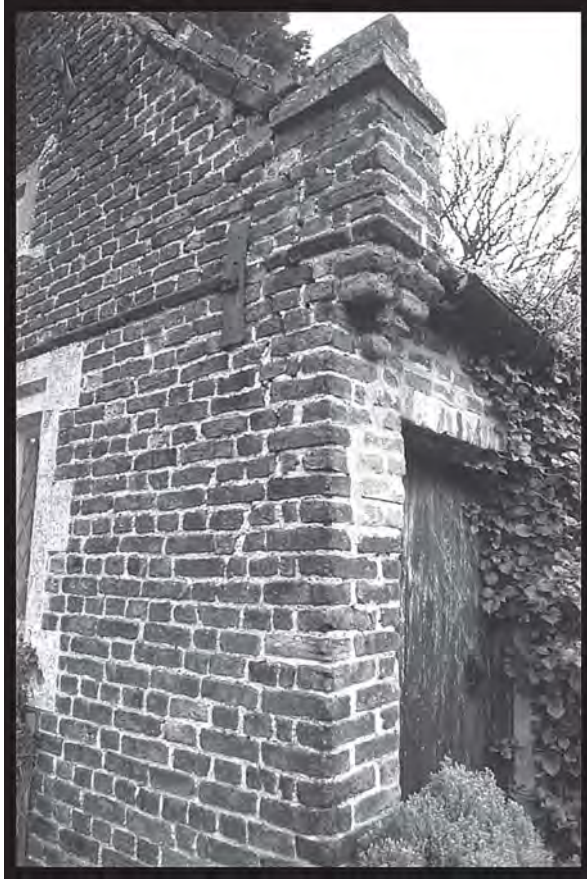
Detail of decorative corbelling supporting a straight parapet on the Little Thurlow Almshouse (1618), Suffolk England. Photograph by Willie Graham, 2001.
