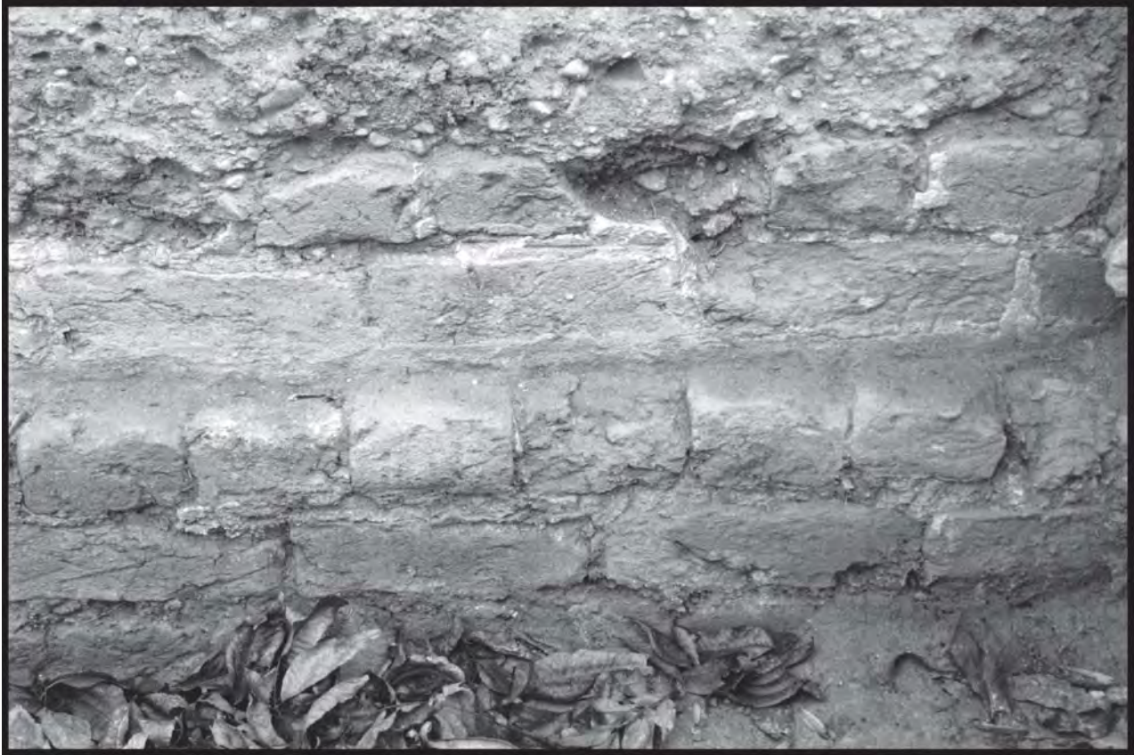
Foundations of House 5, east of west chimney. Note the remains of grapevine joints. Joints were painted with the same red wash as the brickwork, applied before the mortar had dried. Photograph by Carl Lounsbury, 2001.
