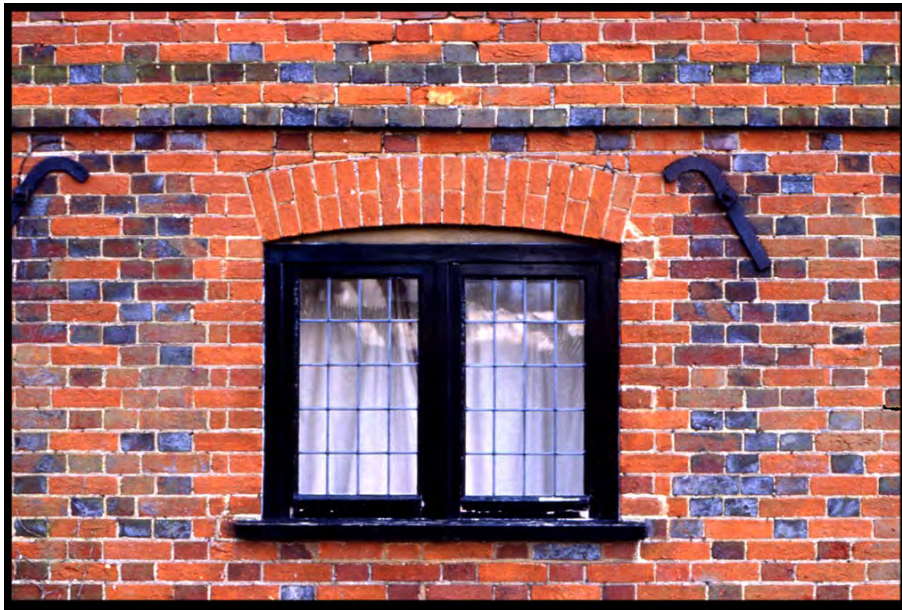
Cottered Almshouse (ca. 1700). By the end of the seventeenth century, masons were skilled in the use of manipulating color in brick walls. Note the lighter, rubbed work around the window and the decorative placement of glazing in the wall and stringcourse. Photograph by Willie Graham, 1994.
