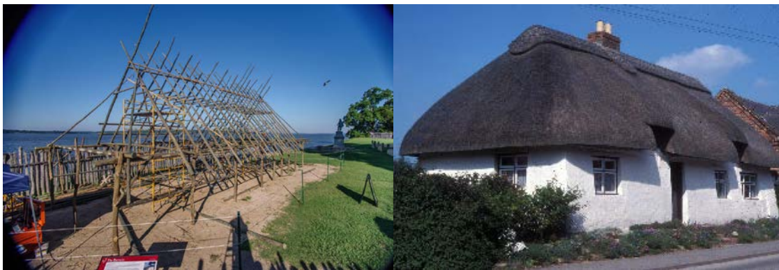
(Left: 2020 barracks reconstruction project underway. Right: “mud-and- stud” style building in Lincolnshire, England)
